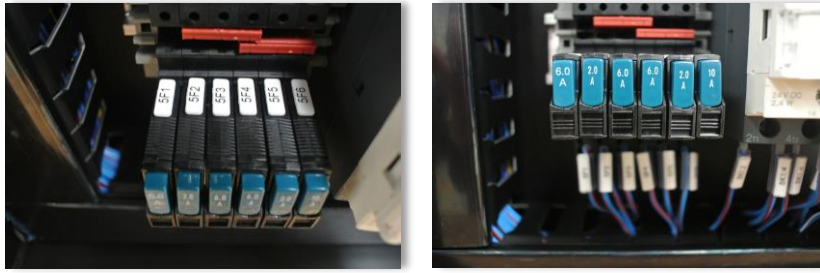
24VDC Circuit Protection Fuses
