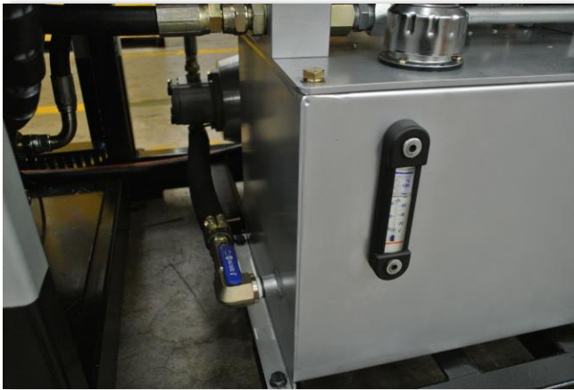
Hydraulic Reservoir Fill Cap and Sight Glass
